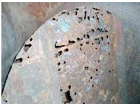
Holes in fire damper
