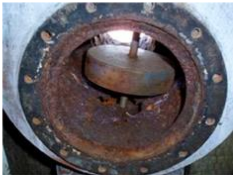
Ballast tank head vent on a ship is rusted and not working.
