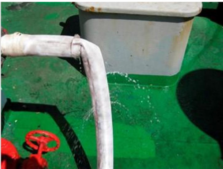
Fire hose that is attached on a ship. It has holes and water is leaking out
